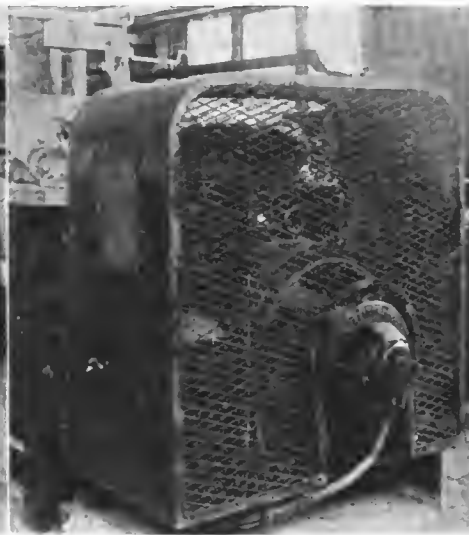
Another expanded metal and sheet iron guard for covering motors, starting boxes and switches, making it impossible for either workers or material to touch them
